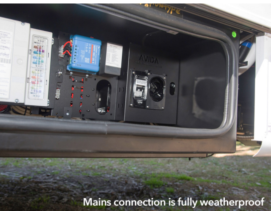
Externally stored AGM batteries
